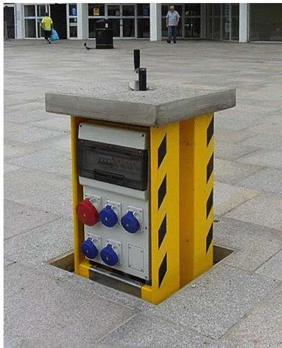
Retractable service units provide access to permanent utilities for temporary events while preserving usable public space when lowered.
